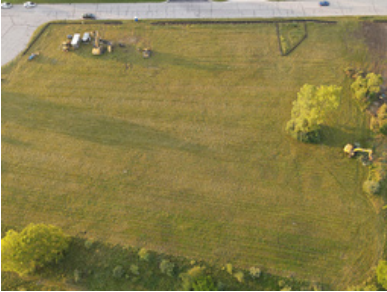
Future Home of Hornet Operations Center, including Transportation and Buildings & Grounds Departments. 1255 Tefft Ct., Saline Industrial Park
